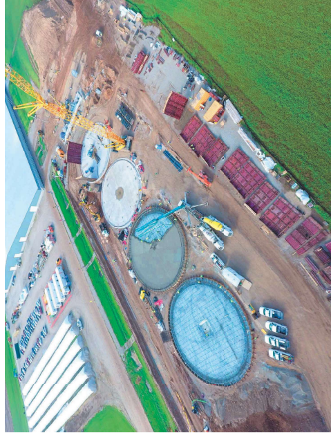
RNG project under construction – imagine trying to do 70 of these in the next year
